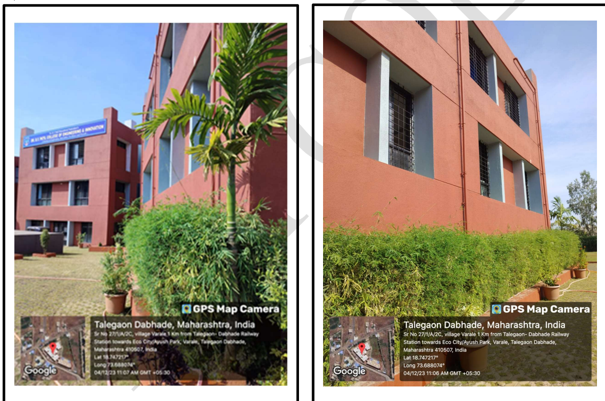
Down Pipelines to collect and drain roof top water for ground recharging at Dr. D. Y. Patil College of Engineering & Innovation
